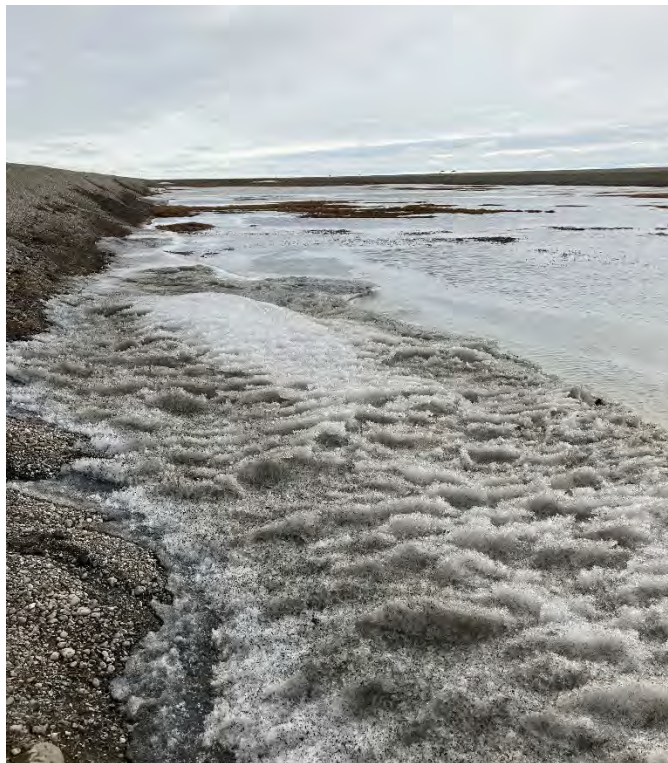
Exhibit 1 - Snow and ice in drainage ditches (facing east).
