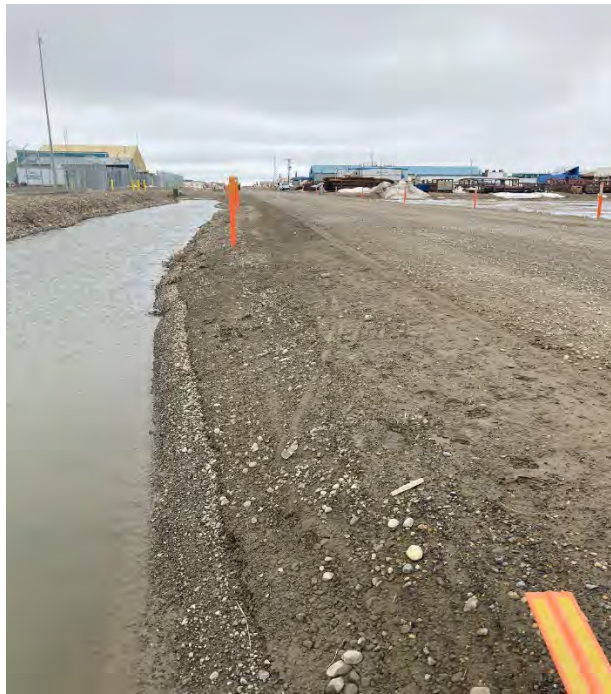
Exhibit 1 - Standing water in the drainage ditches (facing west).
